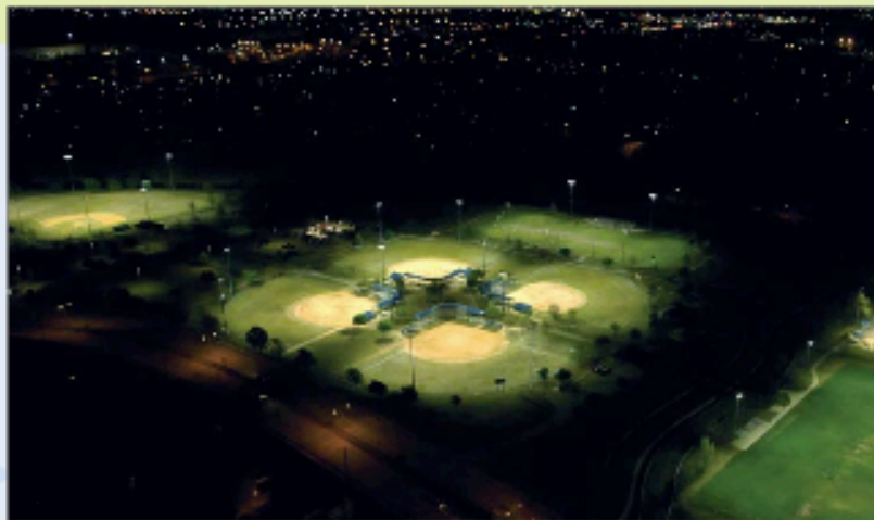
Carrollton replaced a total of 1,838 fixtures on sports fields throughout the city
