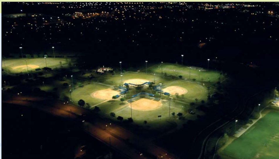
Carrollton replaced a total of 1,838 fixtures on sports fields throughout the city
